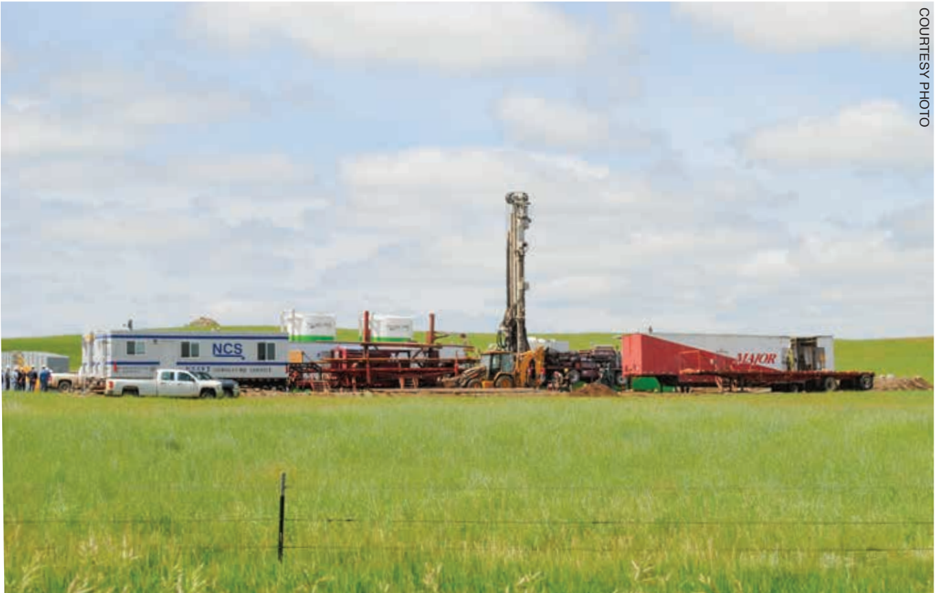
The drilling rig is shown during the operation. The site is about nine miles east and a mile north of Linton.
